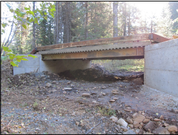
Phillips Bridge over Beaver Creek in Umatilla County. The bridge is designed to improve fish passage.
